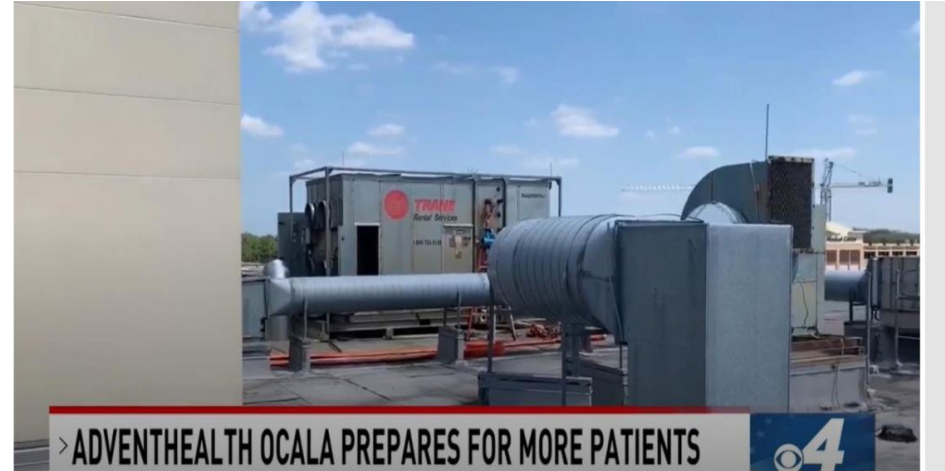
Temporary Once-Through Air/Preconditioned Outside Air Unit
